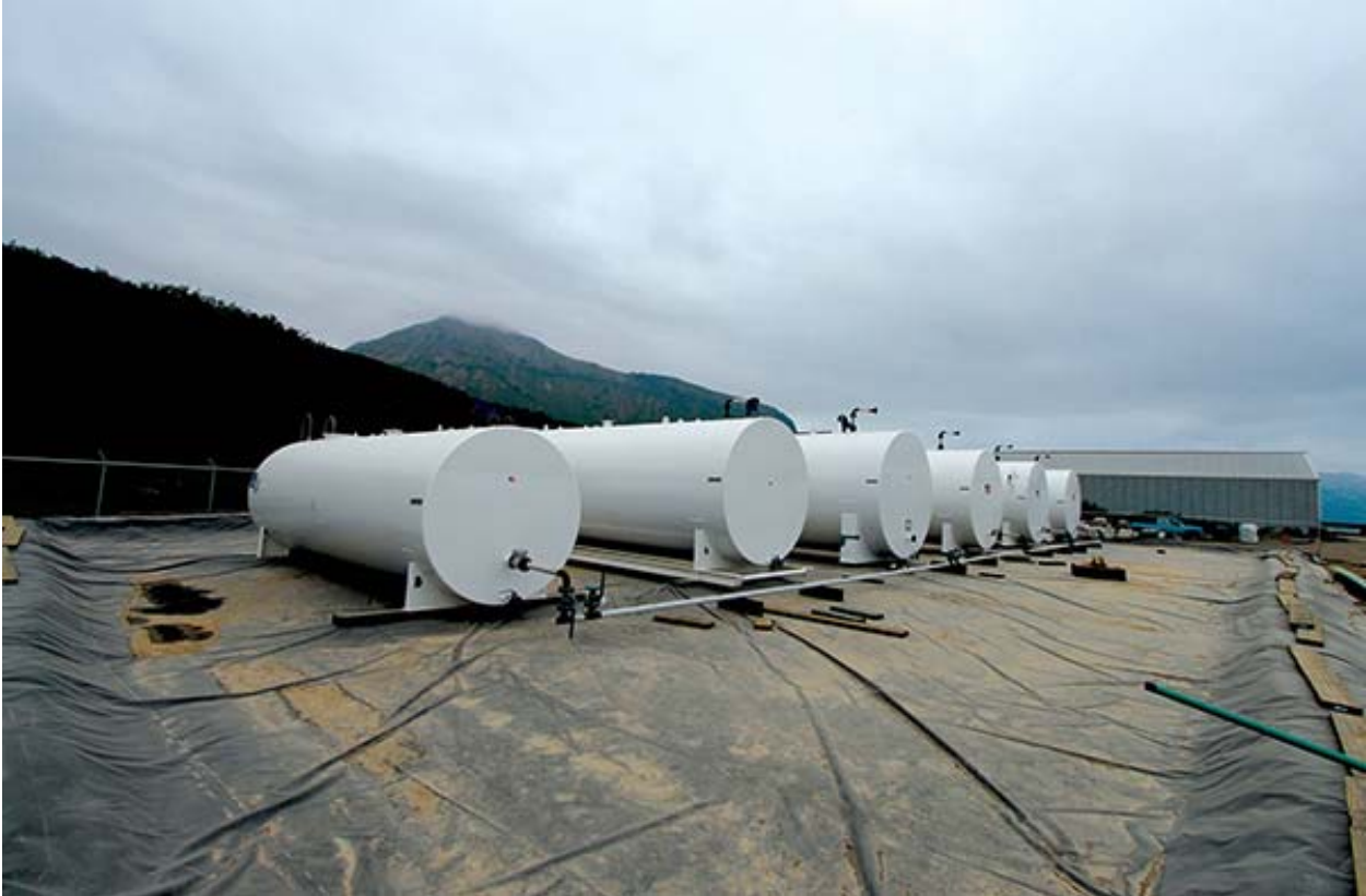
Jpeg photo attached of False Pass Fuel Company storage tanks. Photo credit: Aleutian Pribilof Island Community Development Association (APICDA)
